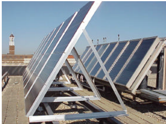
FIGURE. I 3 kW Photovoltaic Array and 30,000 Btu/hr Solar Heating
